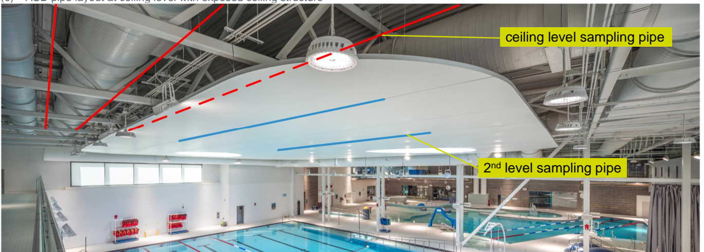
(d) ASD pipe layout at ceiling level with suspended roof structure and additional 2 nd level sampling pipes
