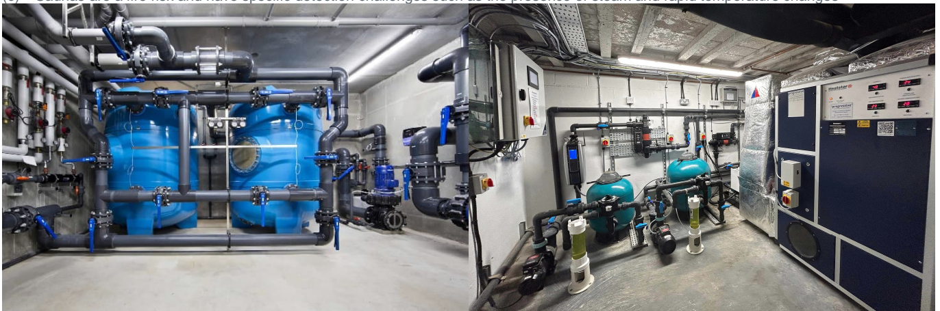
(d) Plant or boiler rooms typically found in the basement of a recreation centre with indoor swimming pool
