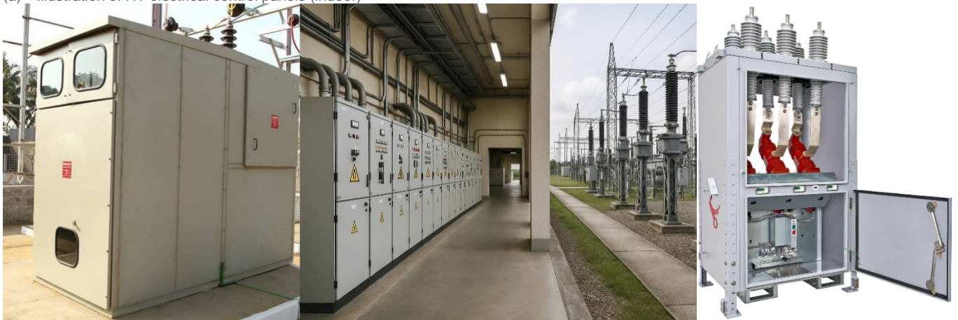
(b) Illustration of HT electrical control panels (outdoor)
