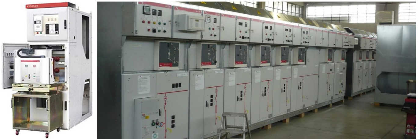
(a) Illustration of HT electrical control panels (indoor)
