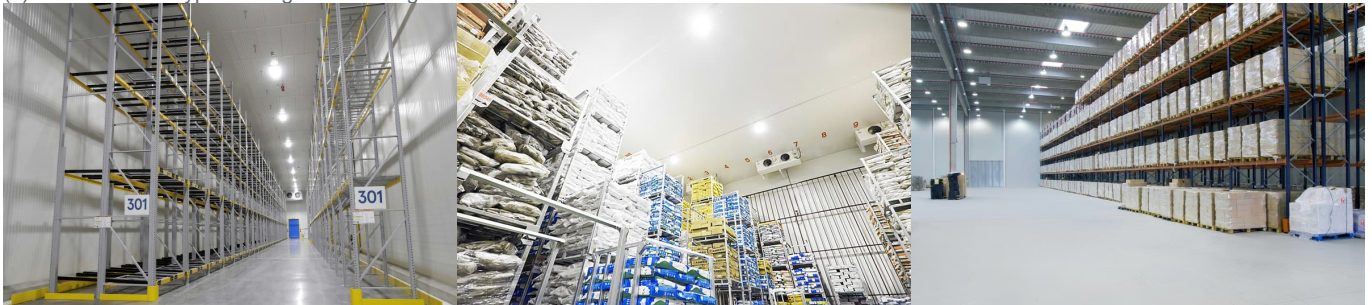
(b) Large open space deep freezers with pallet racks and high-bay storage
