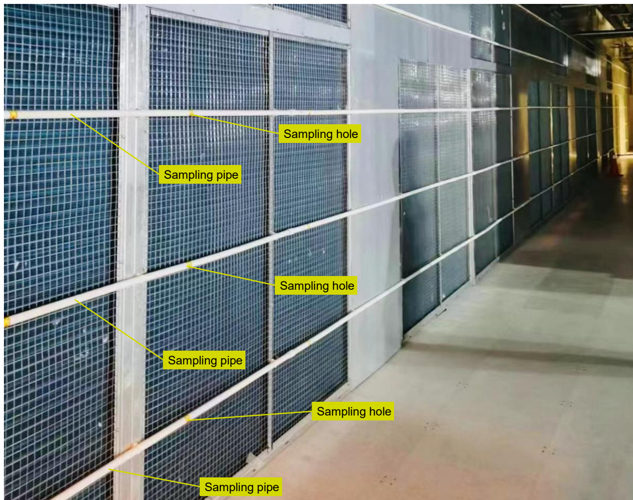
(c) SecuriSmoke ASD pipes covering large return air grill in FAB facility Figure 9 Fire detection placement (duct or exhaust detection)
