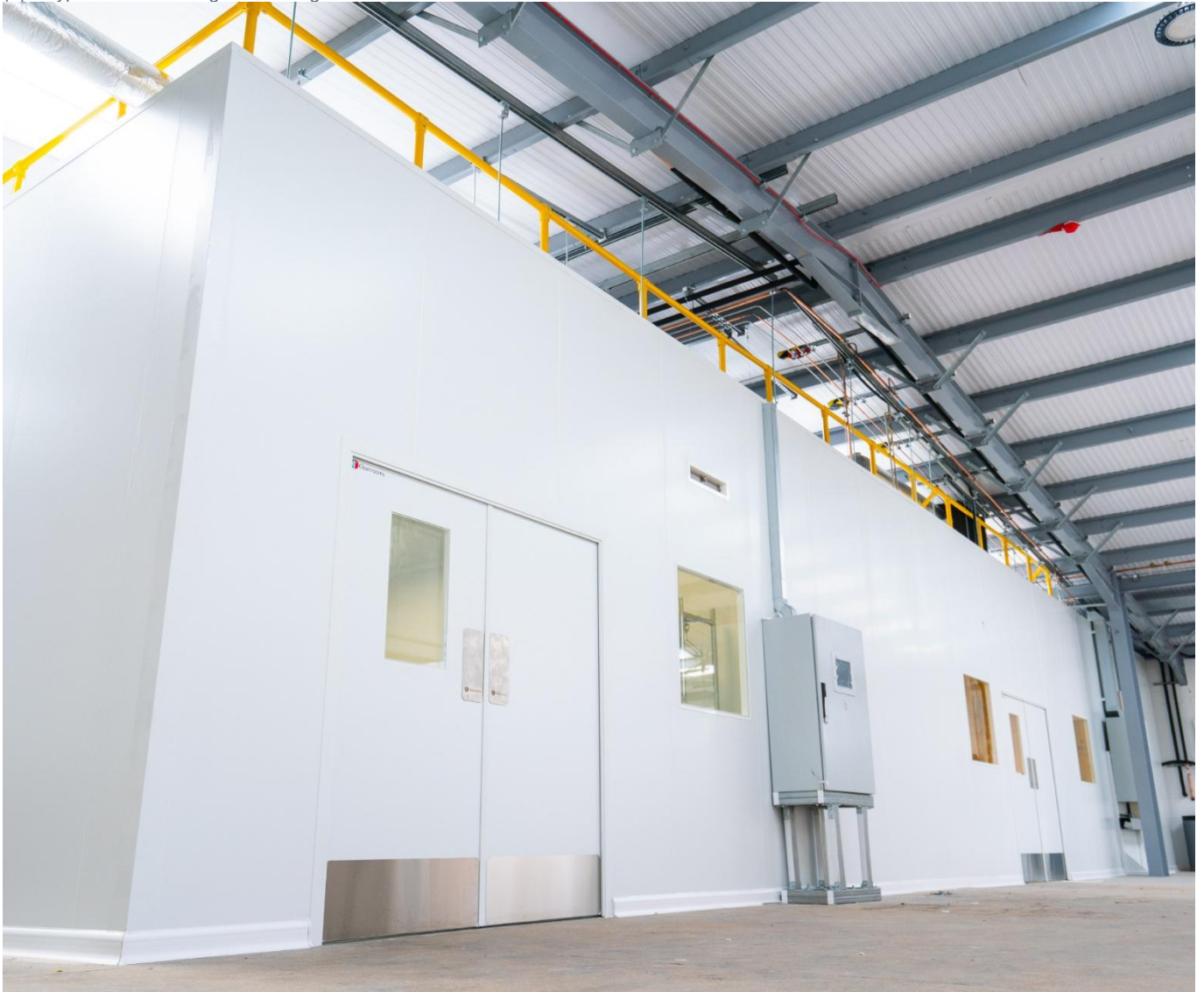
(b) Modular cleanrooms installed within a warehouse-type facility Figure 1 Controlled environments and modular cleanrooms
