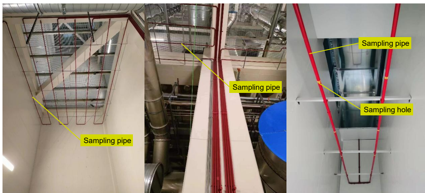
(b) Examples of SecuriSmoke pipe networks installed in FAB and sub-FAB facilities
